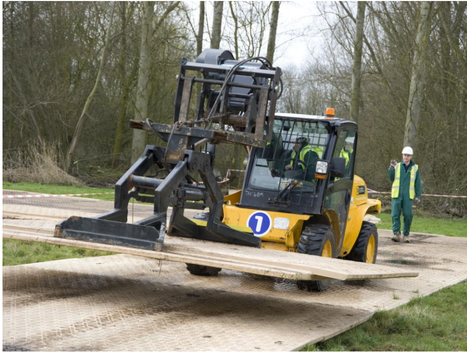
Fig 2 Always use a crew member as banksman. Full PPE must be worn, hard hat, safety glasses, overalls, safety boots, gloves and high visibility waist coat or jacket.
